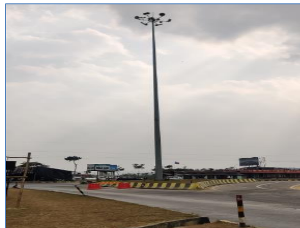
High mast lighting near km 48.600
