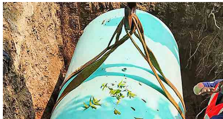
Bio Digester Tank at UEPL
